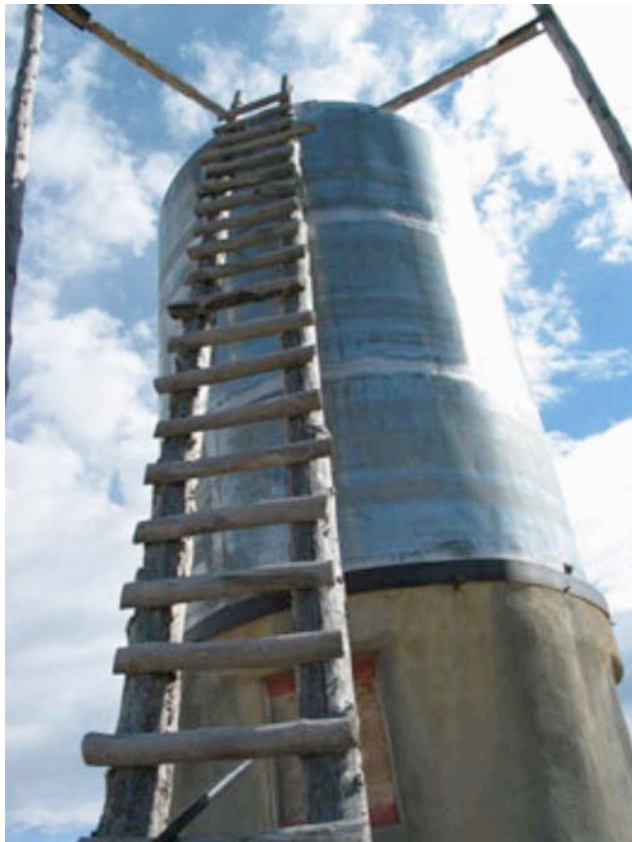
Figure 11 10,000 Gallon Water Tank
